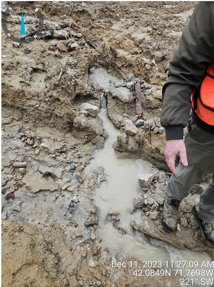
5. Erosion of overburden soils down to, and into, glacial hardpan (north corner of site)
